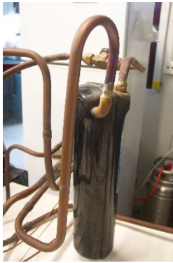
Figure 10. Tank-Accumulator before the compressor
